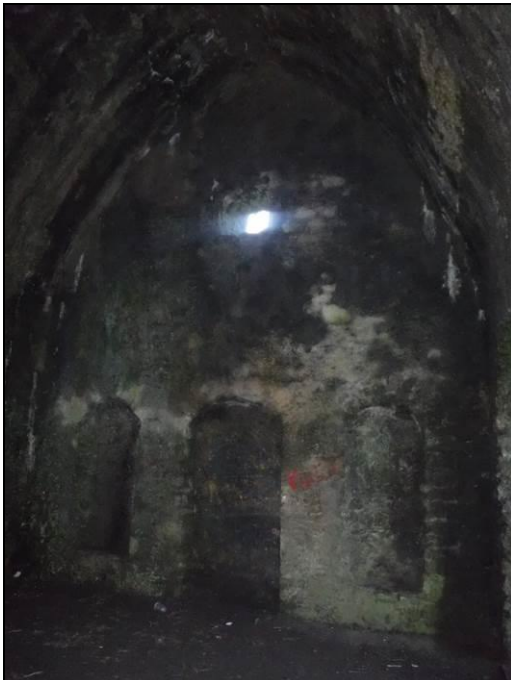
Figure 12.15 The apses in the west wall of the west room on the first floor. The window above relates to the second floor as there would have been a timber floor in between and a vaulted stone roof above.
